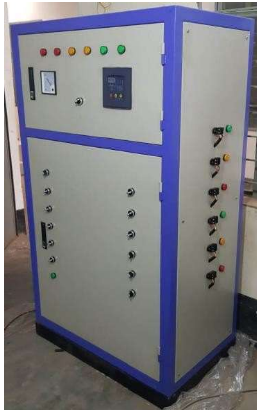
Distribution Panel with PFI
